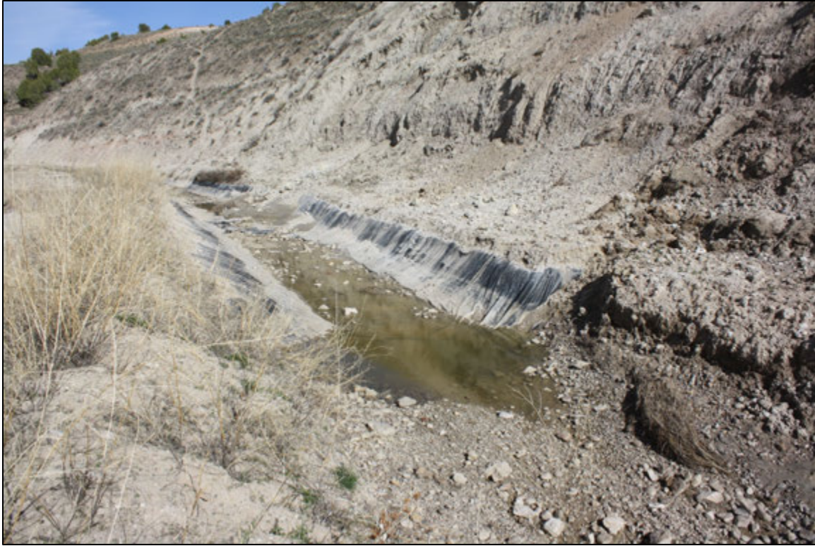
Photo 5. Maybell Canal overview, previously lined portion, view to the east. Note the erosion above the ditch.
