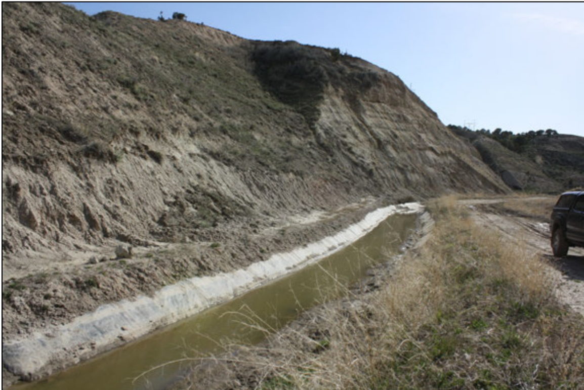
Photo 8. Maybell Canal overview, easternmost extent of previously lined portion, view to the southwest.
